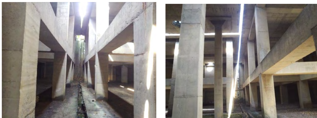
Figure 7 The severe expansion of extension joint
