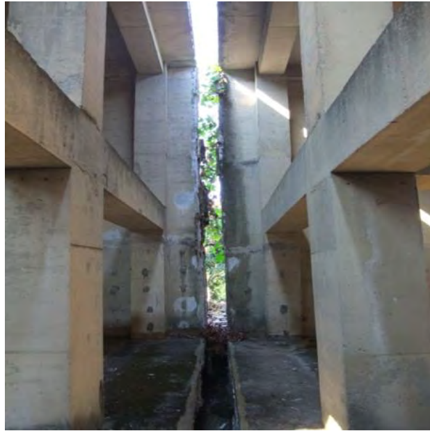
Figure 3 Split of basin from expansion joint
