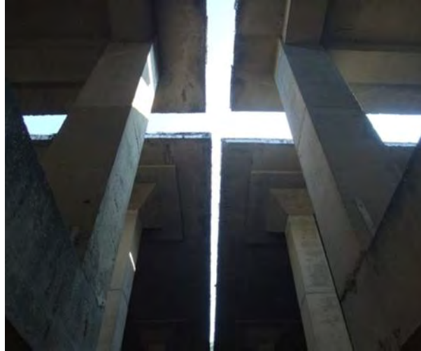
Figure 1 Split of top slab from expansion joint
