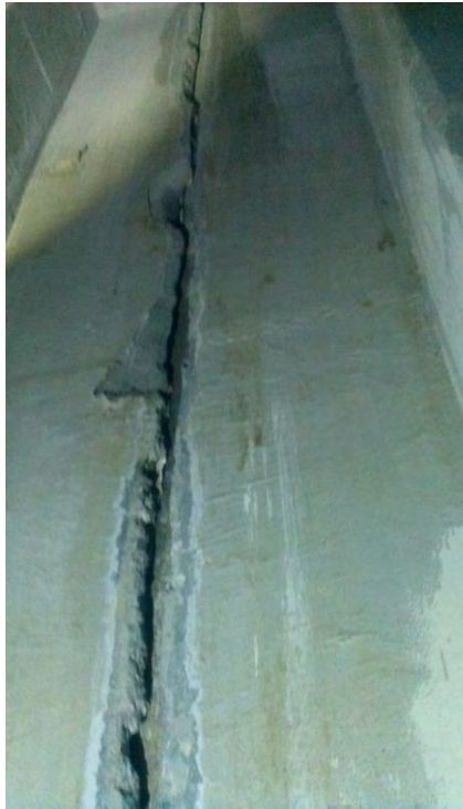
Figure 5 the crack of wall
