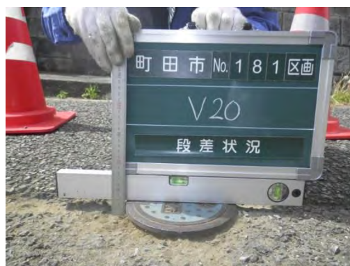
Picture-4: condition of difference in level
