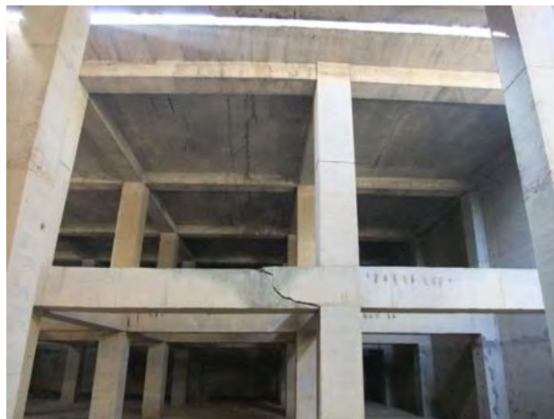
Figure 2 Break in the joint of beam-column joint
